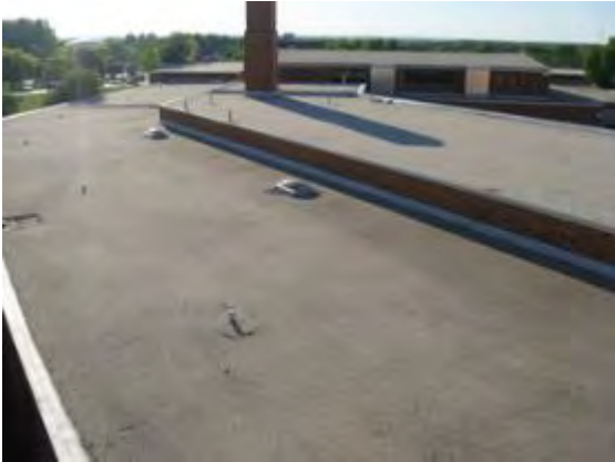
Roofs in poor condition
