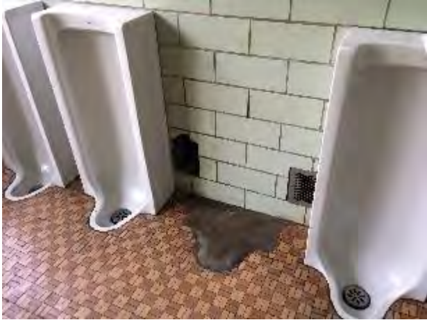
Fixtures in disrepair
