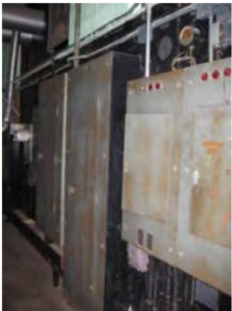
Electrical system is original and in poor condition
