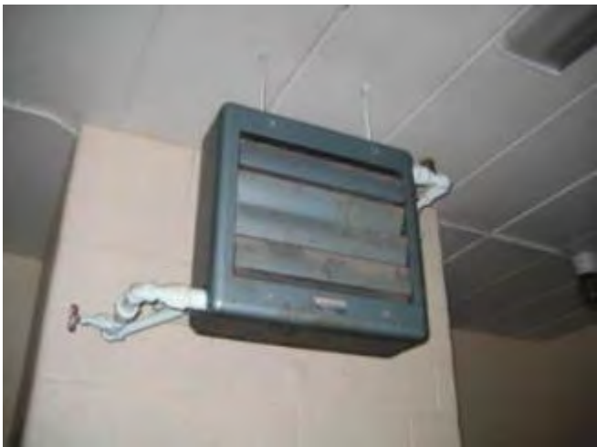
No A/C and outdated Heating / Ventilation System
