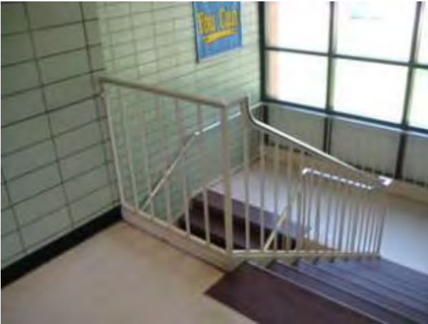
Guard/handrails not Code compliant
