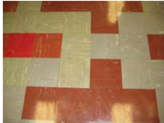
VAT flooring in CR's
