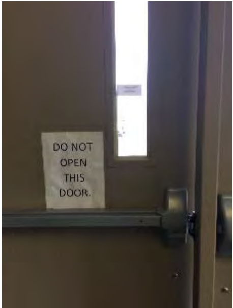
Exterior doors in Poor condition
