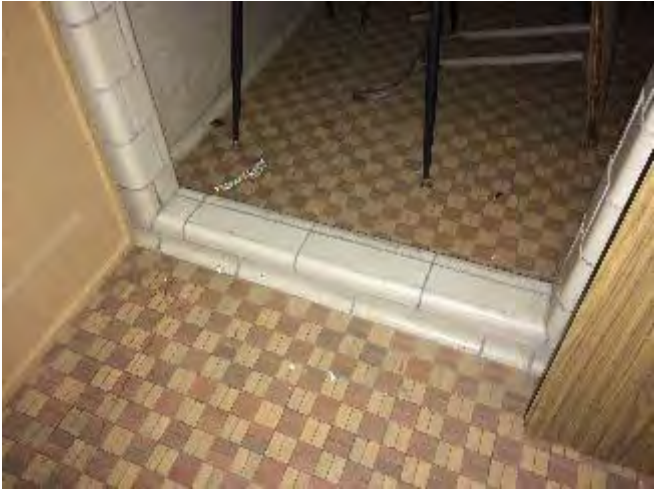
ADA barriers present
