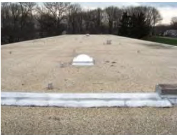
Roofs have multiple layers and some in worn condition
