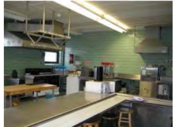
Kitchen & general finishes dated/worn
