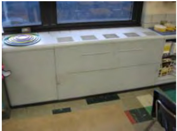
Unit Ventilators do not provide code required amounts of fresh air
