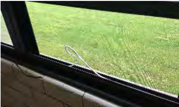
Window gaskets failing
